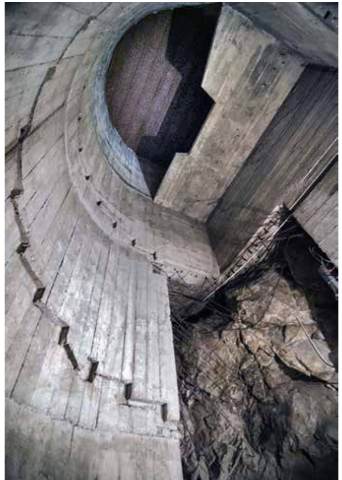
The unfinished ‘D’-shaped stairwell that leads to the tunnels beneath Castle Ksiaz. Photo Mike Scott
